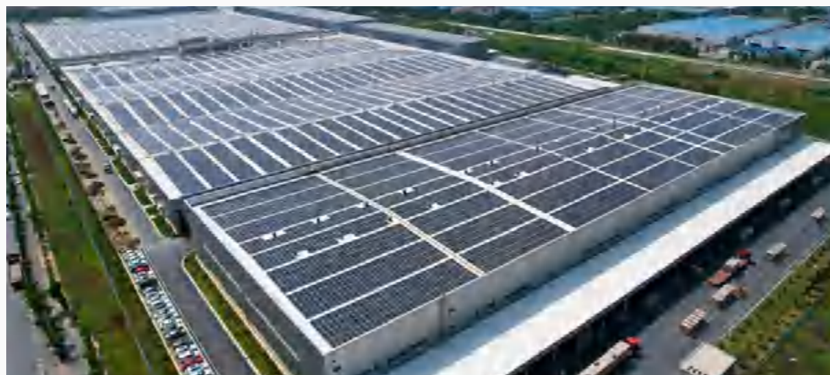
Hefei GCL SI Xinyu PV Power Station
